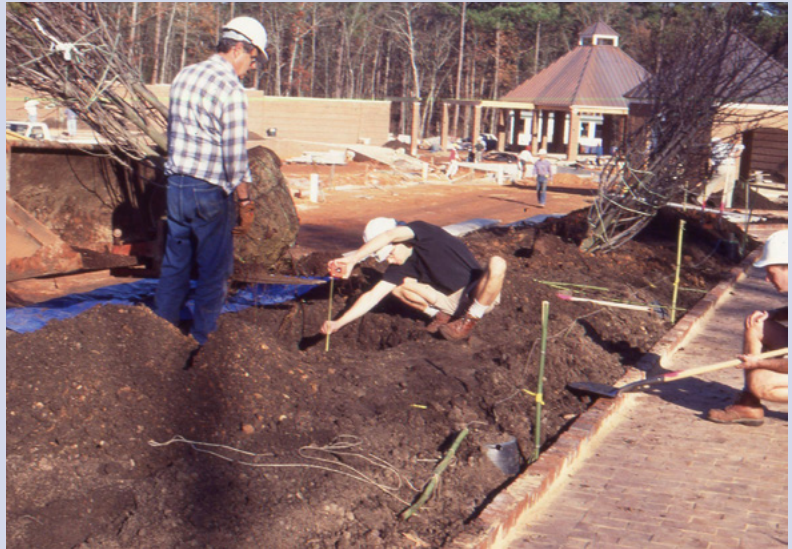
Young Jenks and Tommy Cave precisely planting trees on the Garden construction site in 1991.
